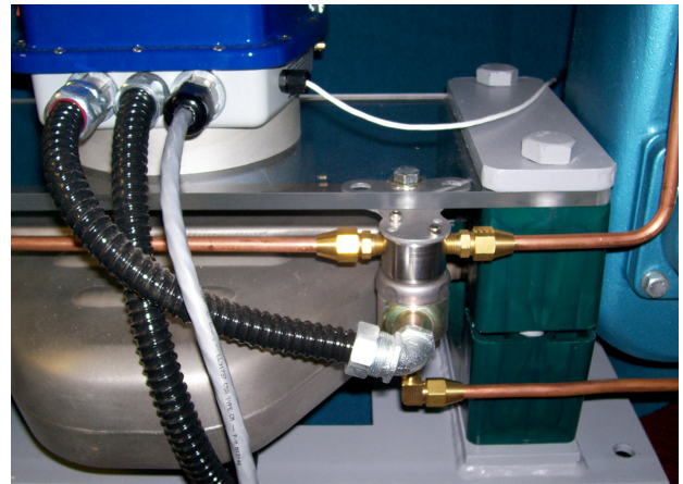
Figure 4-9. Valve Wiring and Plumbing
